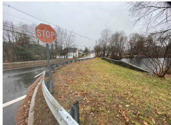
The guardrail along the Shaw Conservation Area presents a significant barrier to even informal pedestrian activity, and the large curb radius further exacerbates walkability issues.
